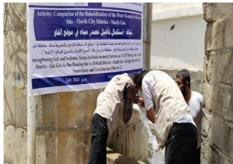
Rehabilitation of the well at Western Al-Faw site and pumping fresh water for the IDPs
